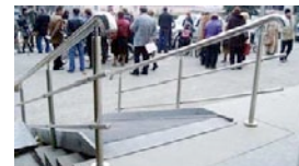
Figure 5. A steep ramp, with a slope greater than 1:12, illustrating an inaccessible entrance.
